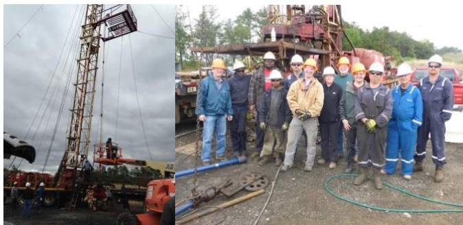
Figure 2: (Left) Operations during bio-mineralization sealing of a well at the Gorgas Powerplant (AL). (Right) Field crew after successful well sealing.
